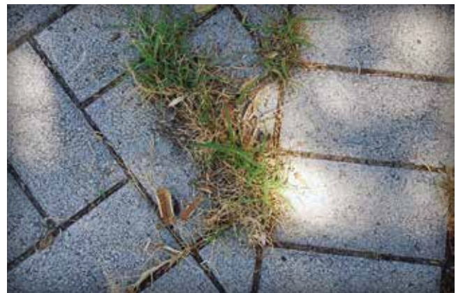
Figure 9. Weeds indicate sediment accumulation and lack of surface cleaning to remove it.
